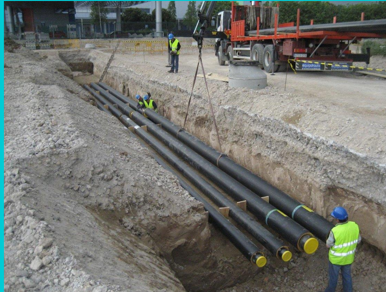
Photo: Pipes for data center district heating in Stockholm. Fair use.
